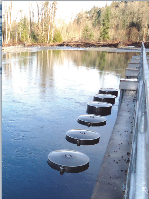
Elwha Surface Water Intake Screens
