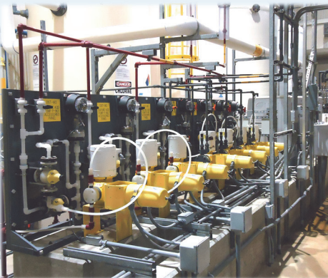
Chemical Storage & Pumps
